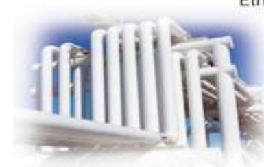
Industrial Gases Pipeline
